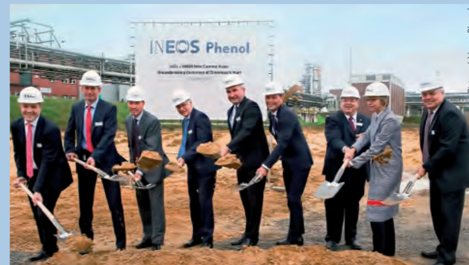
Ground-breaking ceremony for one of the world's largest cumene plants being built for Ineos Phenol at Marl
